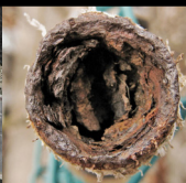
Pipes are rusting
