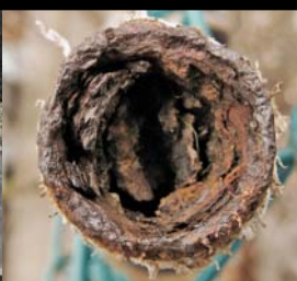
Pipes are rusting
