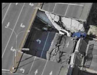
Roads are crumbling
