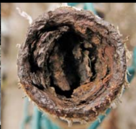
Pipes are rusting
